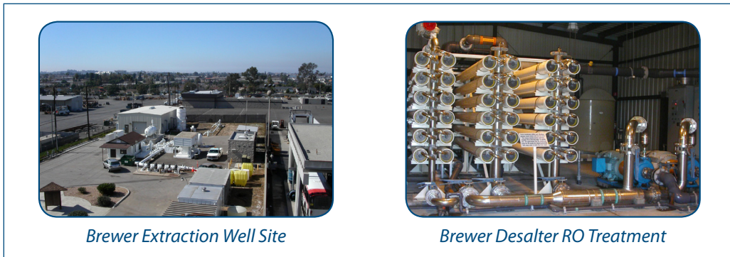
Figure 10-4: Brewer Desalter Facility Equipment
